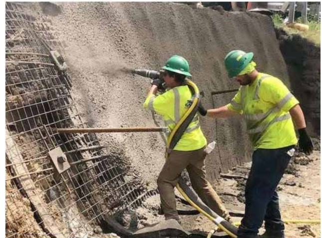
Fig 8: Application of shotcrete layer over prepared diaphragm wall surface using compressed air spraying equipment.
