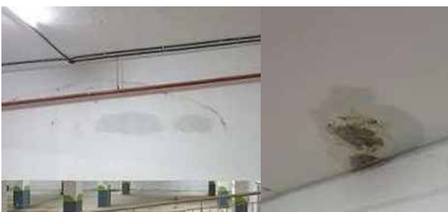
Fig 2: Water oozing out from the retaining walls
