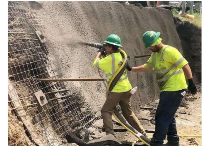
Fig 8: Application of shotcrete layer over prepared diaphragm wall surface using compressed air spraying equipment.
