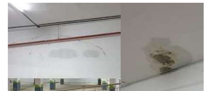
Fig 2: Water oozing out from the retaining walls
